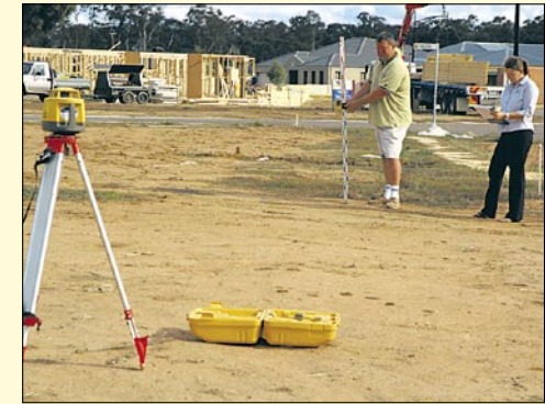
Darren Pitt, Construction Manager and Kellie Aveyard, Sales Consultant conduct a preliminary site inspection for a client, which includes taking levels to determine site fall.
